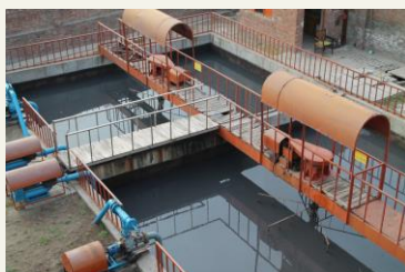
Wastewater treatment in Lahore tannery ©WWF-Pakistan
