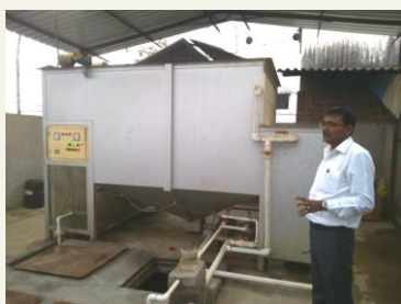
Effluent treatment plant in Moradabad metalware factory ©WWF-UK/Conor Linstead
